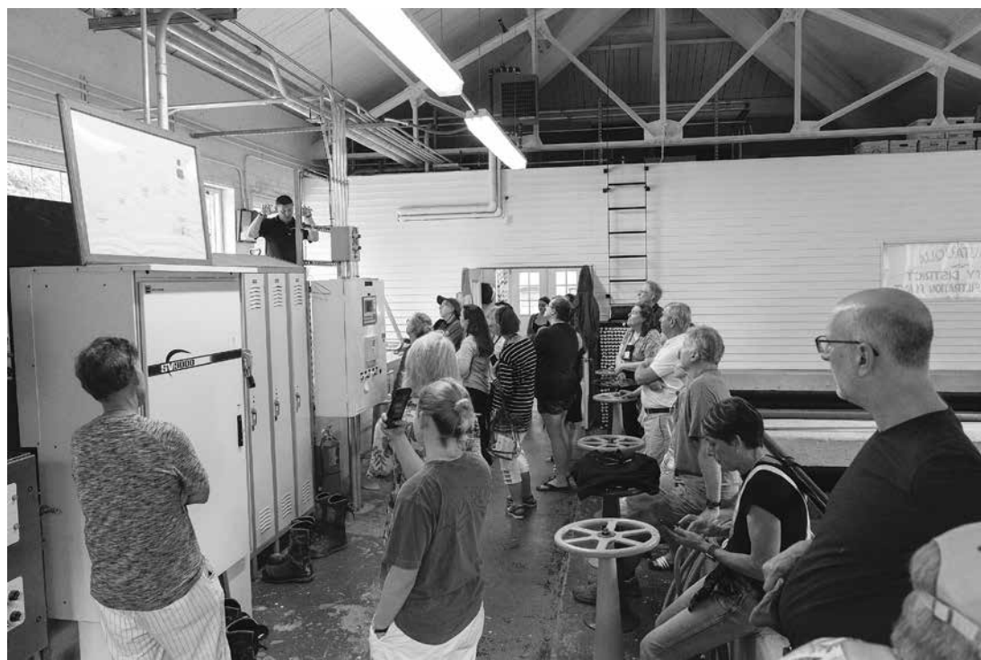
Chautauqua Utility District Superintendent Mike Starks gives Chautauquans a tour of CUD's Water Filtration Plant last Monday.
